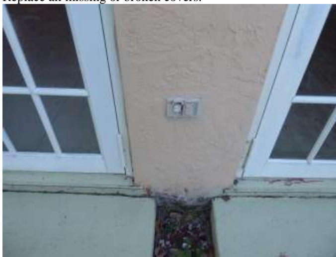
Broken conduit at A/C condensing unit, wiring is exposed.
