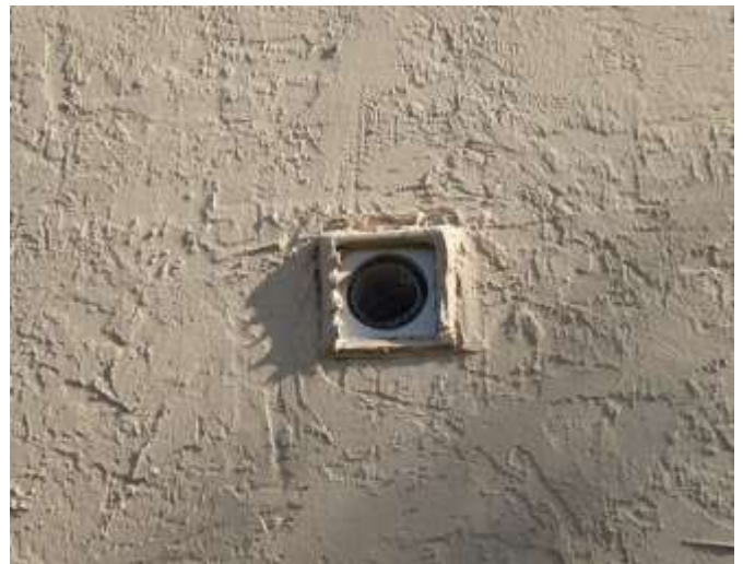
First floor bathroom exhaust hood.
