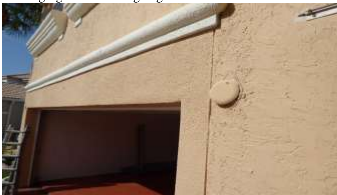
Inoperable light fixture at 1st floor hallway and exterior flood lights.
