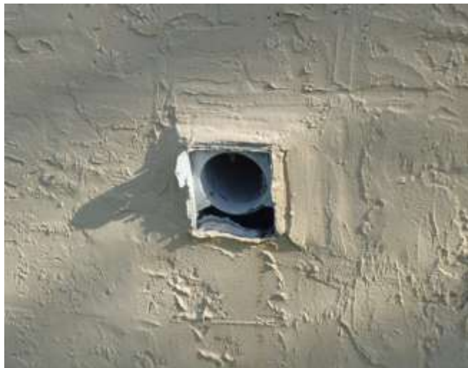
Dryer exhaust hood
